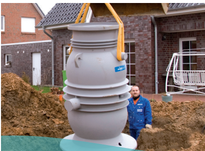
Pressure drainage plants
