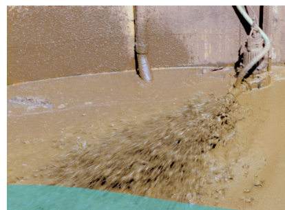
Liquid manure pumps
